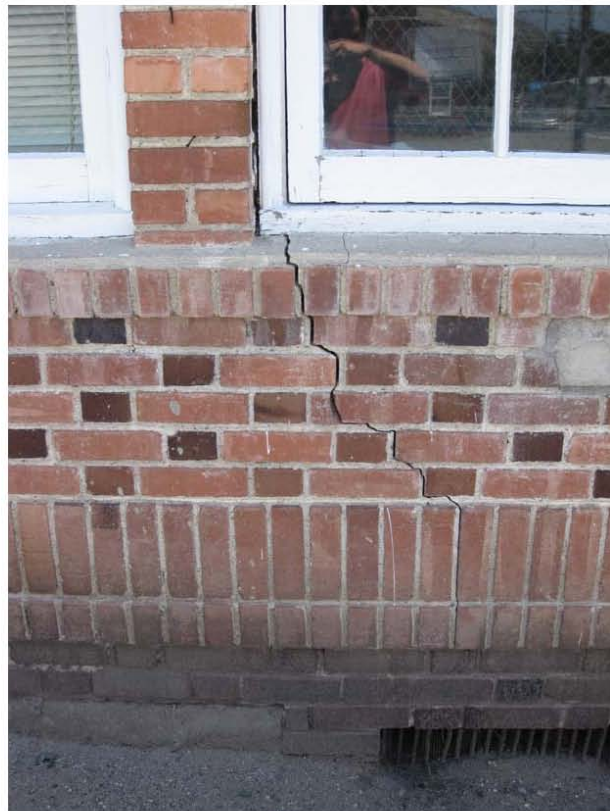
Figure 5 – Crack Near Southwest Corner
