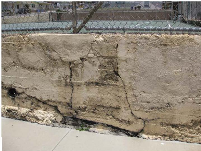
Figure 7 – Cracks in Tennis Court Wall
