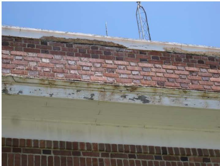
Figure 4 – Spalling Concrete and Exposed Rebar at Cornice
