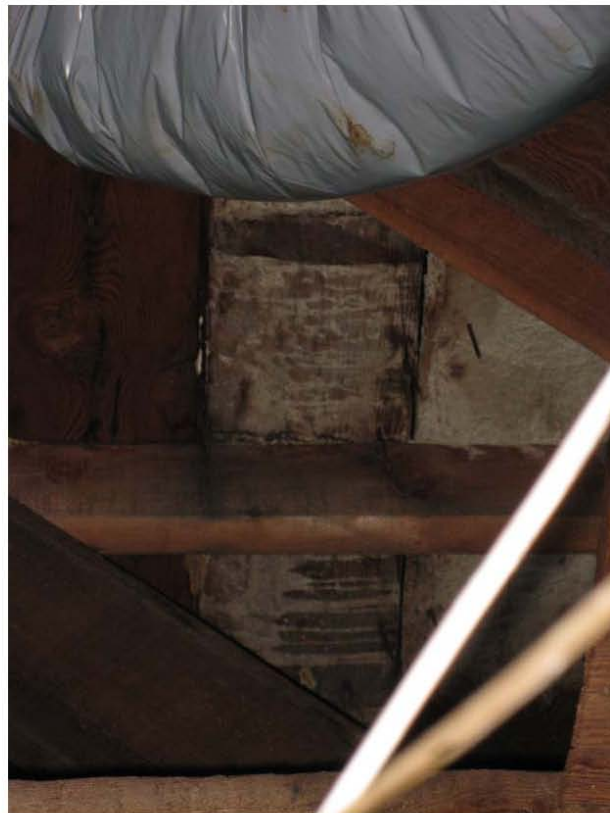
Figure 1 – Mold and Dry Rot at Roof Framing
