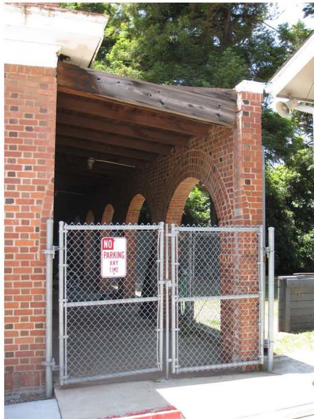
Figure 6 – Location of Previously Removed Damaged Arch
